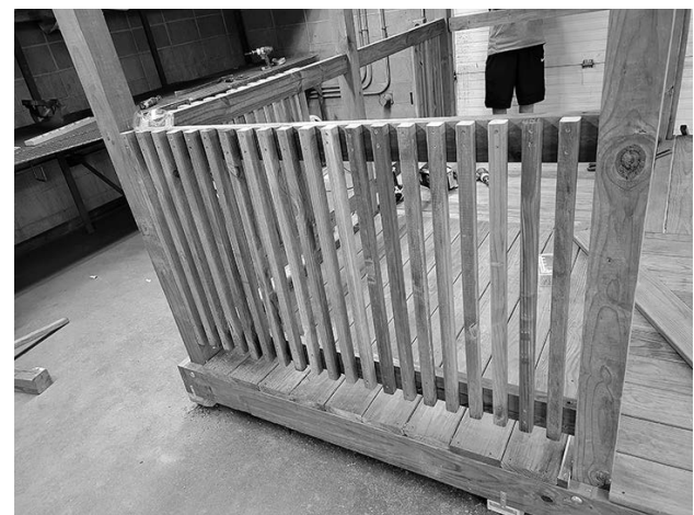
This picture shows the current part of the project the Ag Construction students are working on, which is installing the railing of the gazebo.
